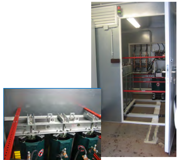
MOBILE MEDIUMVOLTAGE RAP (Container)
