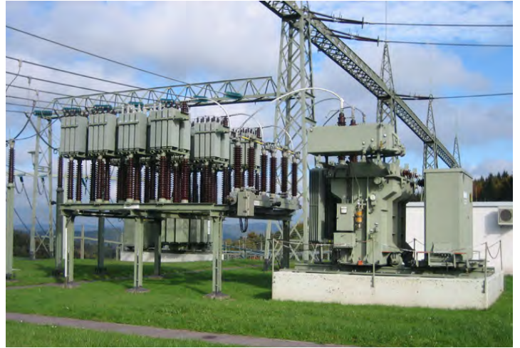
HIGHVOLTAGE RAP 110kV (Outdoor)
